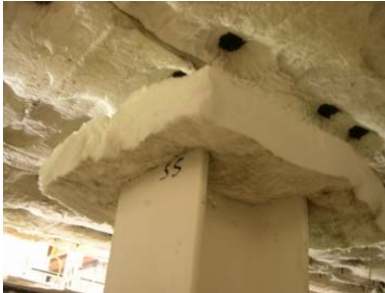
Column tops insulated with ceramic blanket and pressed against the furnace lid
