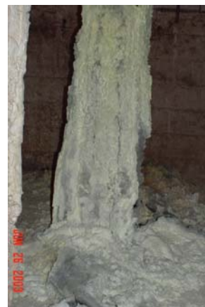
#12: Bottom of column after test.
